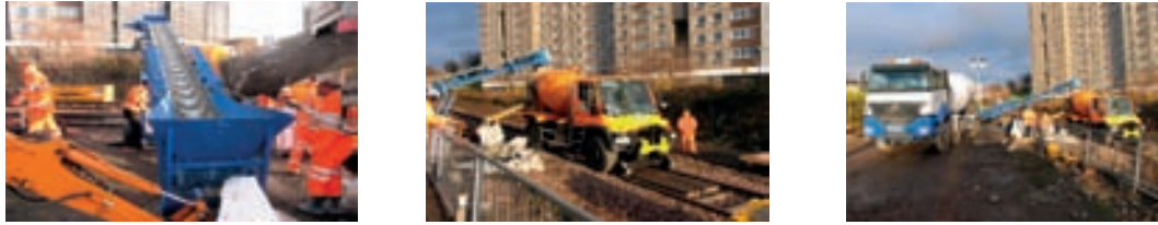
Figures above illustrate discharge onto conveyor, which filled a 3m 3 rail-mounted small truck mixer
