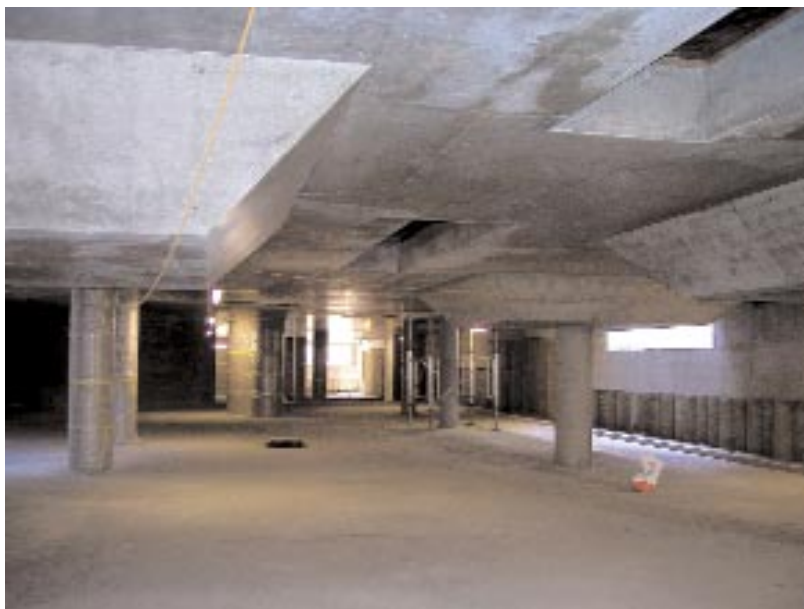
Figure 2: A plywood layout was used on the soffit to provide accurately aligned joints in the basement car park.
